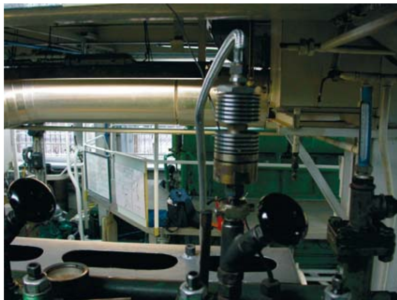
Fig. 2. View of pressure sensor PT - 5101E installed on indicator valve of cylinder number 5
